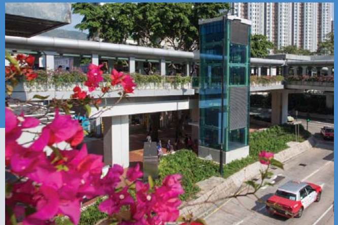
Lift installed at footbridge across Castle Peak Road near Nan Fung Centre, Tsuen Wan
