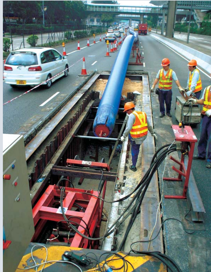
15-year replacement and rehabilitation programme of 3,000 km aged water mains - advanced trenchless technology was adopted to minimise disturbance to the public and traffic
