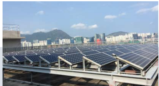
The PV installation in the APB Centre in Hung Hom (Existing building retrofit)
