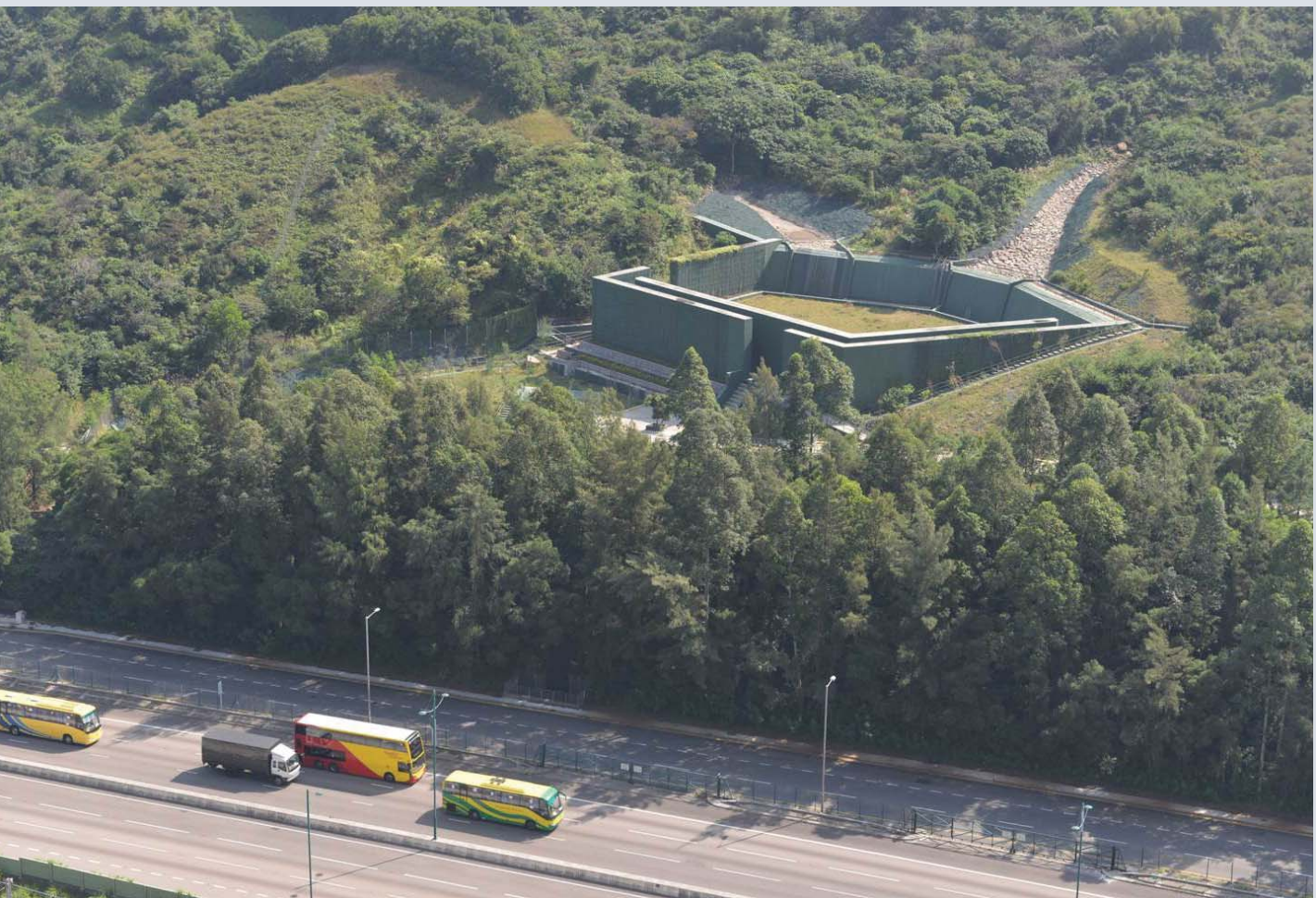
A debris-resisting barrier protecting North Lantau Expressway, the major road-link to the airport, against debris flow
