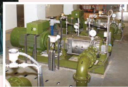
Wah Fu Salt Water Pumping Station
